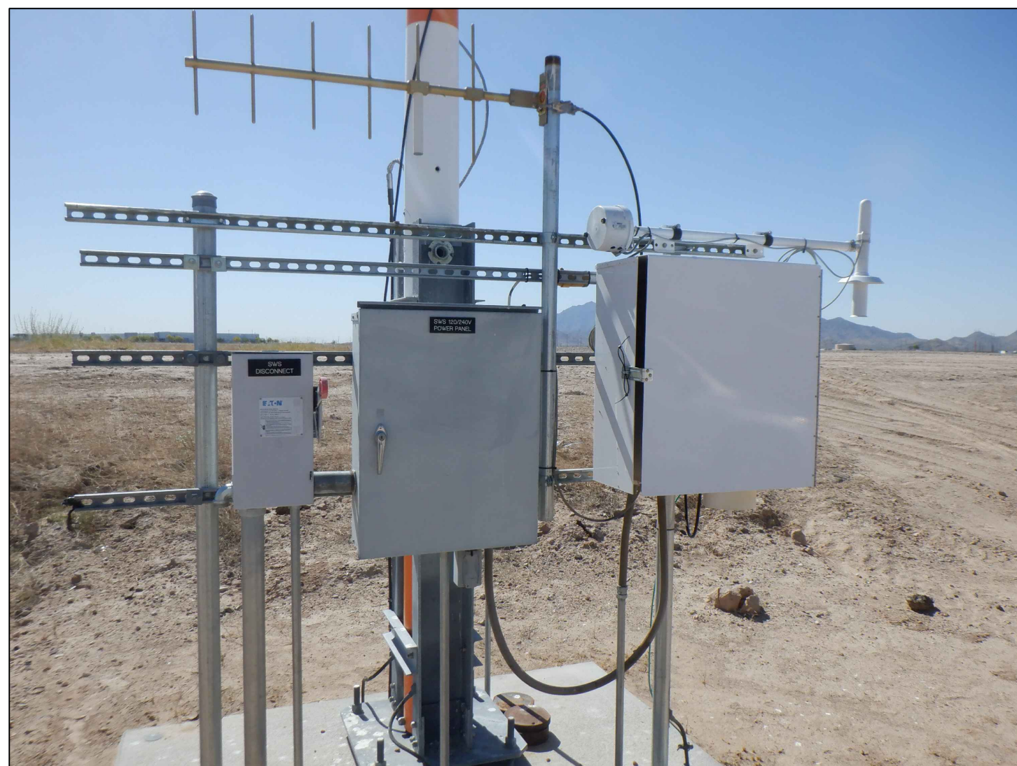
1 TYP EXISTING SWS EQUIPMENT FACING NORTH WEST
