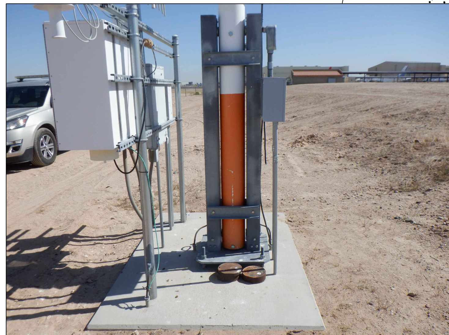
2 TYP EXISTING SWS EQUIPMENT FACING NORTH EAST
